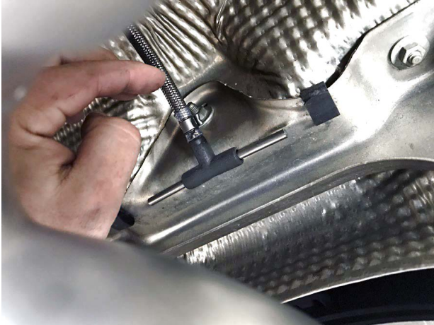
Pictured Left: Vacuum T-Block with both left and right vacuum hoses removed.
