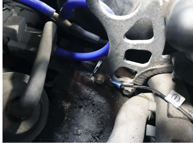
Pictured Left: Crimp eyelet to the ground wire on the valve controller
