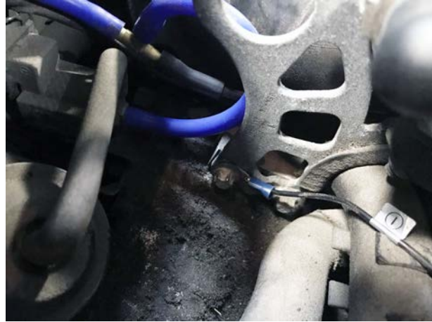
Pictured Left: Crimp eyelet to the ground wire on the valve controller
